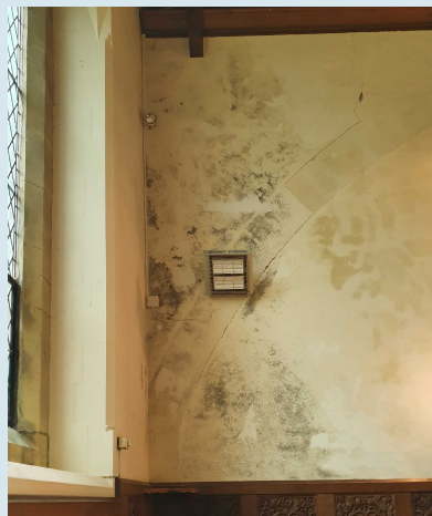
Water ingress in the south transept
